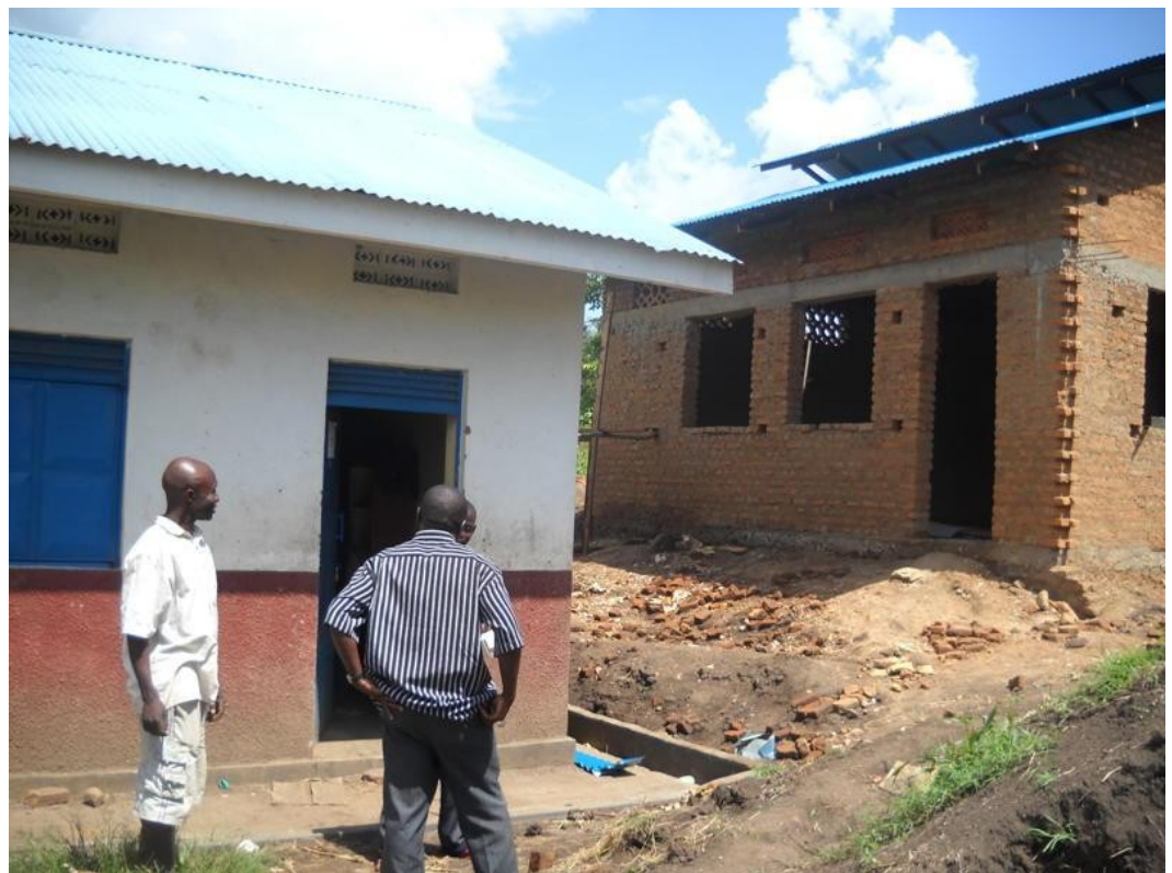
The contractor building the new kitchen at the Primary School, (in white shirt) confers with other KARUDEC staff members. They are standing in front of a dormitory (hostel) for boys.
