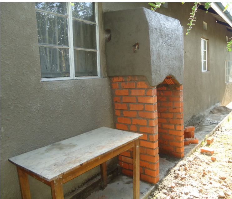
Construction of the water heater in progress. The stainless steel tank is embedded in the fire bricks and fire cement plaster; pipes not yet installed to supply hot water.
